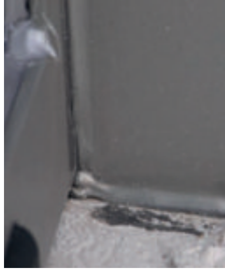
Figure 55.- Scellant incorrect (Source : ASEFAVE)
